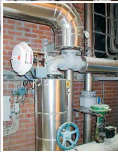
Körting thermocompressor in a paper factory
